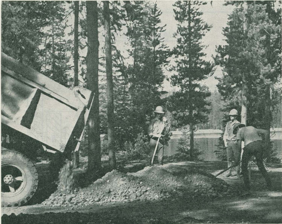
A load of gravel, and this youth crew will soon refurbish this camp-site at Crooked River Park.
