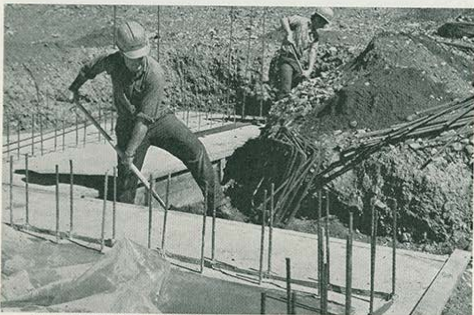
Lower terminal of new chair-lift in the Gibson Pass Ski Area of Manning Provincial Park during early stages of construction in August. The chair-lift was completed and operating by December 1970.
