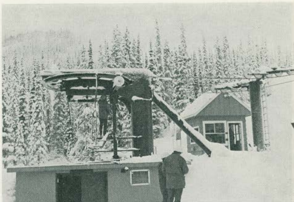
Workmen making final adjustments to Gibson Pass Ski Area Chair-lift No. 2, prior to acceptance for public use.
