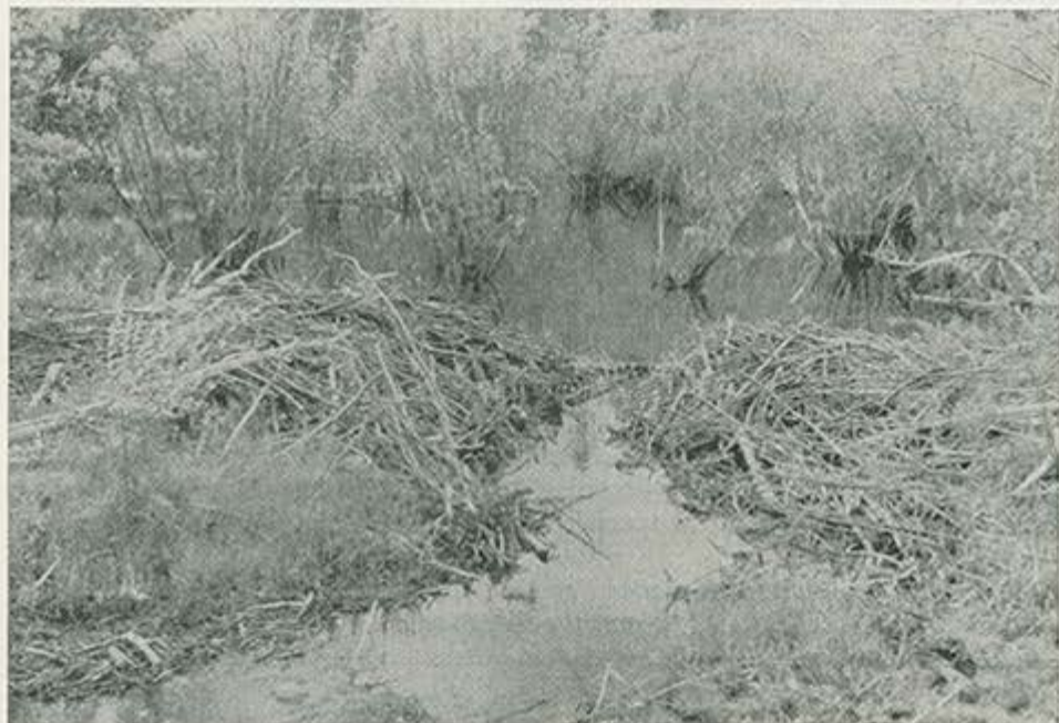
Example of stream obstruction caused by beaver activity.
