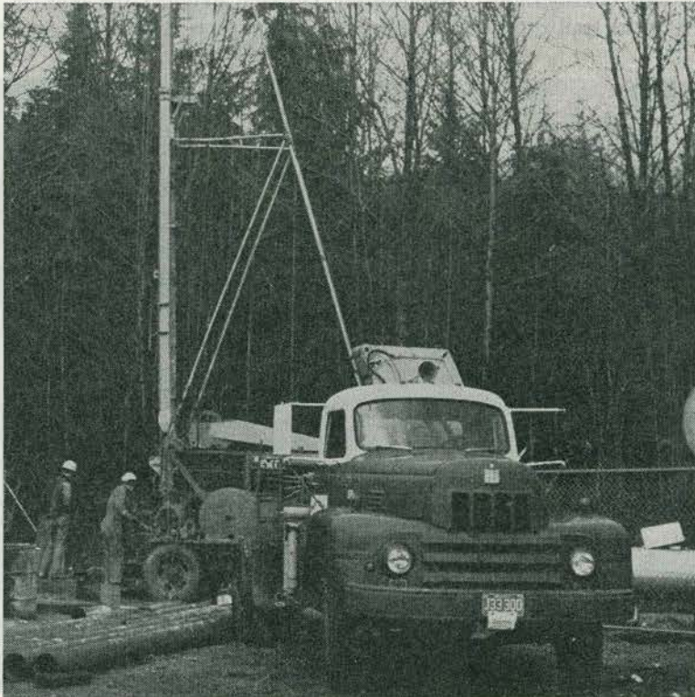
Drilling-rig at Golden Ears Provincial Park—an example of a continuing programme to provide better water systems in the parks.
